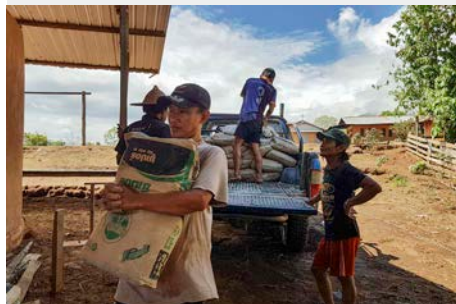
Most materials are from site, but some few must be bought. Paw Eh Wah arranges this
